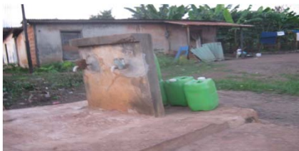
Dry stand pipe in Boadi
