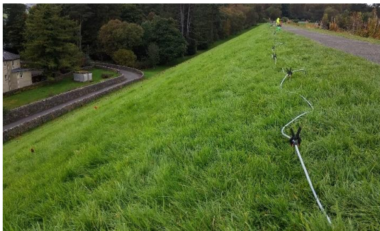
Fig. 3 Views of the crest and the downstream face of Mugdock reservoir dam.
