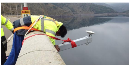
Figure 11: Receiver antenna installation at El Atazar Dam. Intercontrol Levante SA [13]
