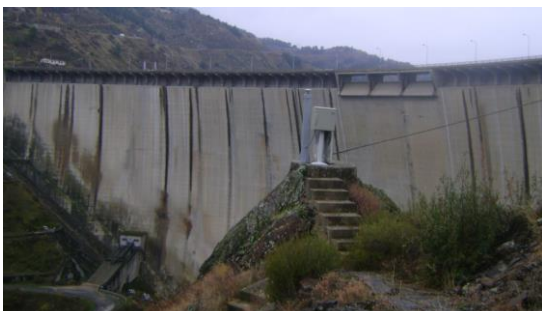
Figure 10: Monitoring station in El Atazar Dam . Intercontrol Levante SA [13]
