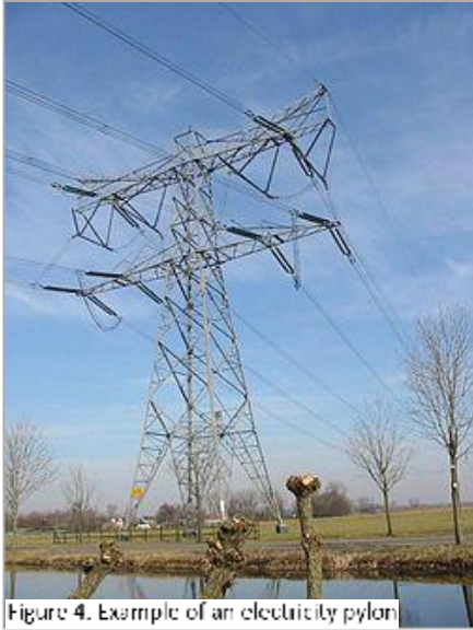
Figure 4. Example of an electricity pylon
